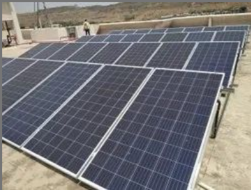
Solar Rooftop On Grid System
