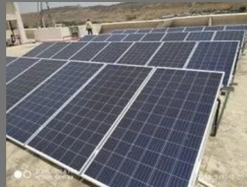
Solar Off Grid System
