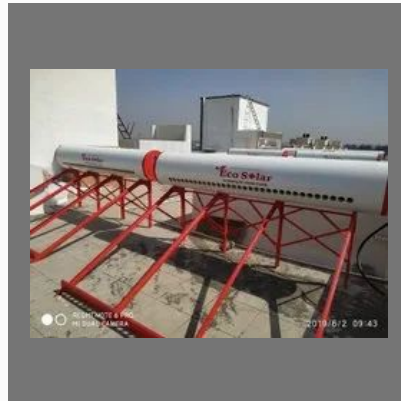
Solar Water Heater Tank
