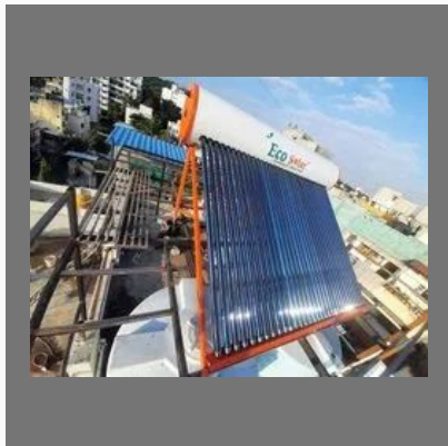
Solar Water Tank
